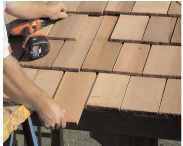
64. Slide first 24" long Filler Shingle where roof panels meet until flush at bottom.
